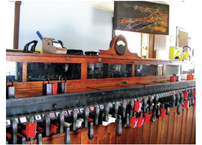
The 80-lever G pistol-grip electric interlocking machine was housed in a large wooden console. A track model board above the console showed the 80 switch locations on each of the railroad tracks.
